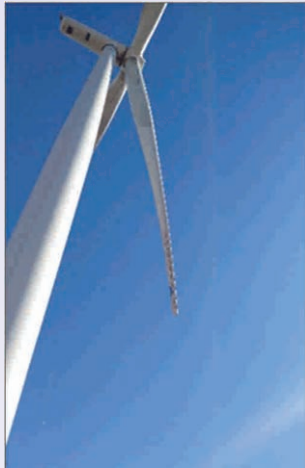
Figure 4: The damaged turbine before application
