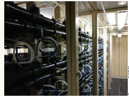
Redox Flow Battery
